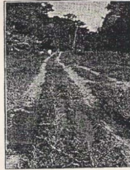
It may not look like much of a road, but this could open up Tortuguero village to considerable expansion
